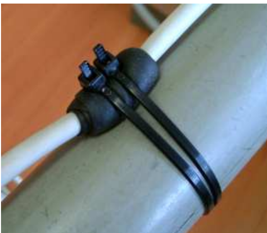
Fig.4.12 Put several layers of self-amalgamic tape around the cable and fix it with cable ties. Usually the cable shield is made from thin aluminum foil which might be cut if the cable is fasten directly tightly with ties without any protection. Also several layers of cloth tape can be used for this purpose. Even UV resistant ties must be replaced after 1-2 years if they are exposed to direct sun light.
